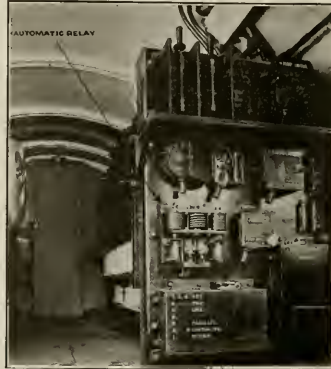
INTERIOR OF CAB SHOWING MAIN SWITCH
